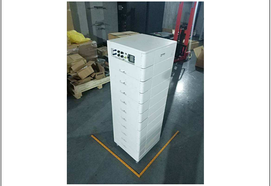
General view-1 of battery
