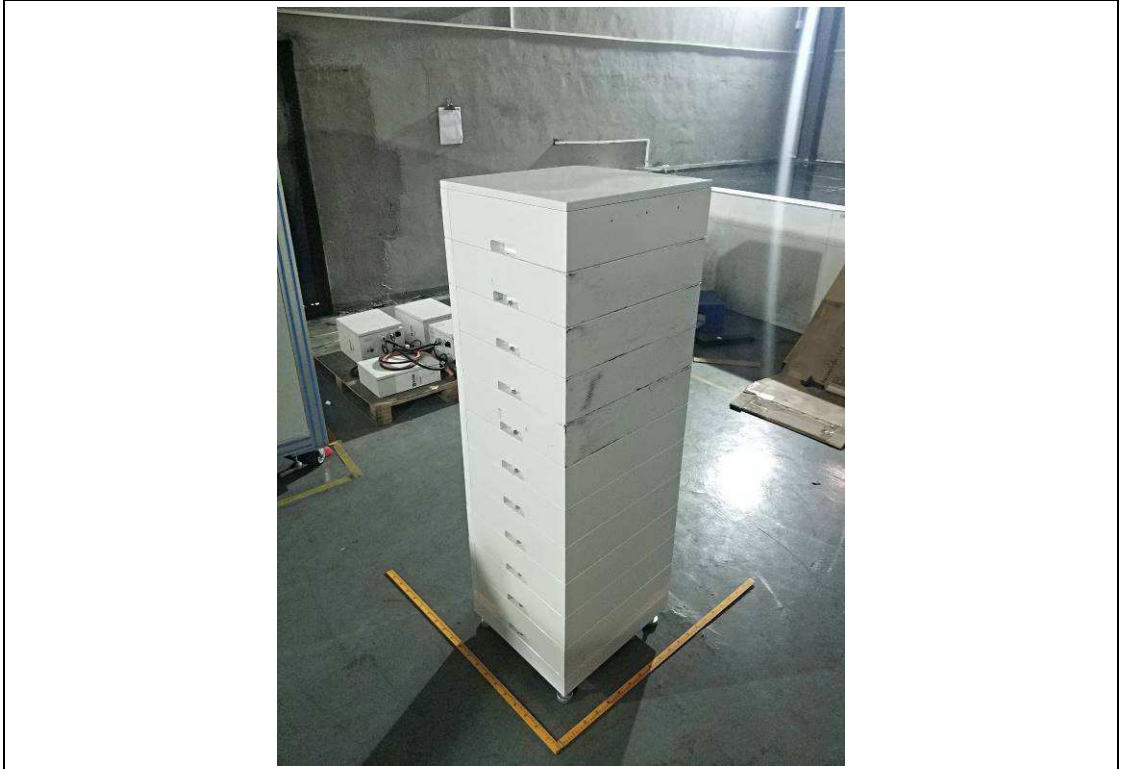
General view-2 of battery
