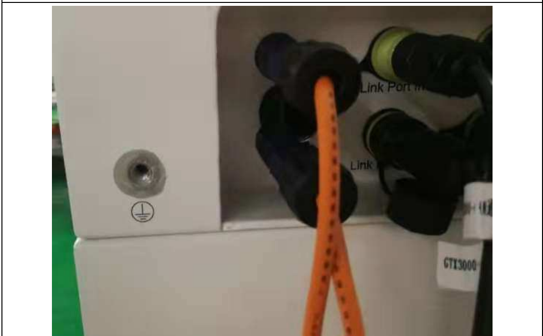
General view of Grounding terminal
